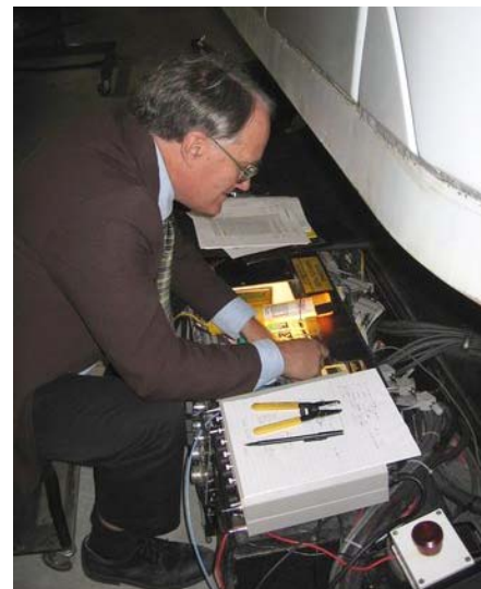
Karl Cunningham, VP of Engineering for Ectron, at work with Model 451 and E408-6Y enclosure.
